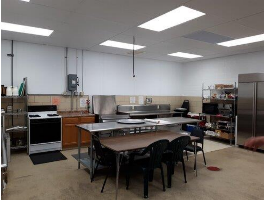
Photo showing completed work in Post 501's kitchen. Much brighter to cook in (June 2020).
