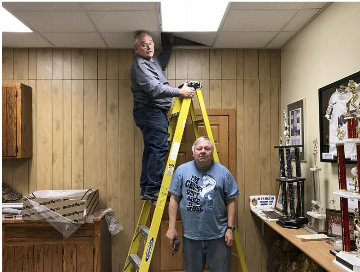
Keith & Jerry installing the last new ceiling tile in Post 501’s Auxiliary & History Room. Well done fellas.
